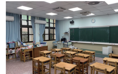
Photo of Completed Installation of LED Lighting Fixtures in the Classroom at Kui Hui Elementary School
